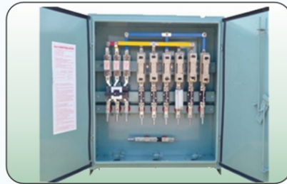
LT distribution box
