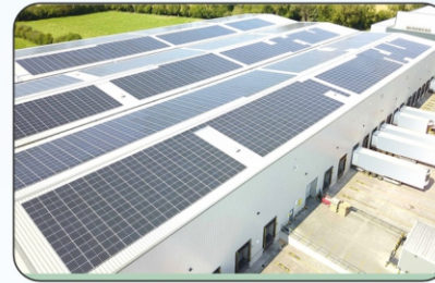
Industrial solar panel system
