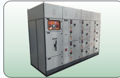
APFC control panel
